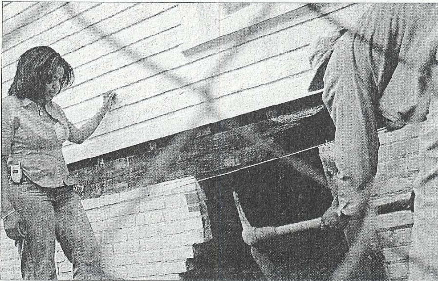
Durham mason William Mack digs into the ground outside one of Realtor Tiffany Elder's latest projects. Elder specializes in restoring and selling old homes in the Durham area.
